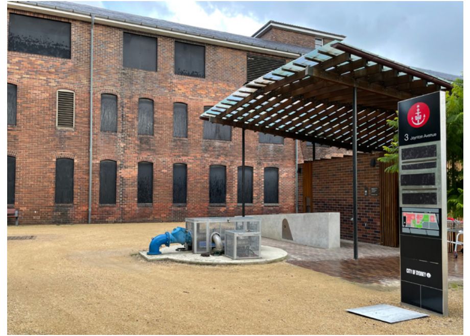
THE WATER REUSE CENTRE, MATRON RUBY GRANT PARK, ZETLAND. PHOTO BY ILARIA VANNI.
