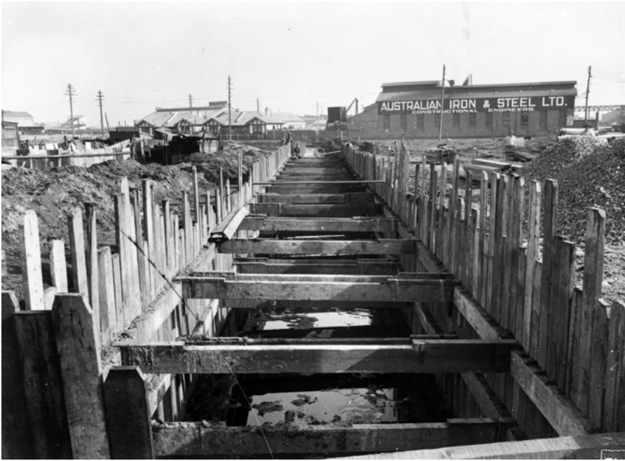
STORM WATER CHANNEL, CORNER OF BOTANY ROAD AND SHIRLEY STREET, ALEXANDRIA, 1929. SYDNEY WATER PHOTOGRAPH COLLECTION, CITY OF SYDNEY ARCHIVES
